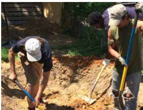
Excavate ~ 2 feet down and add bioretention soil to allow for additional stormwater infiltration.
